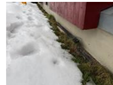
Deformert/vridd topplist langs grunnmur.
