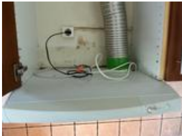
Løse kabler over ventilator.
