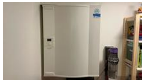
Aggregat plassert i bod.
