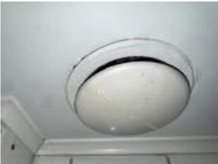
Ventil i himling over toalett.
