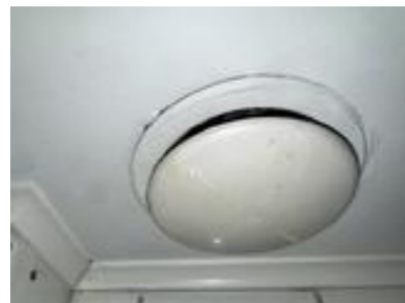
Ventil i himling over toalett.
