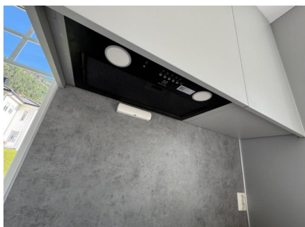
Ventilator over koketopp.
