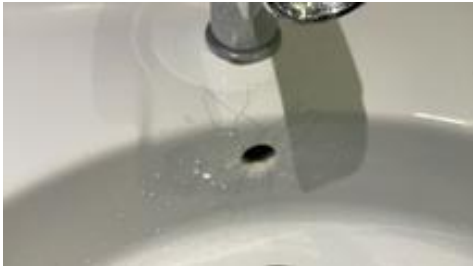
Riss i servant
