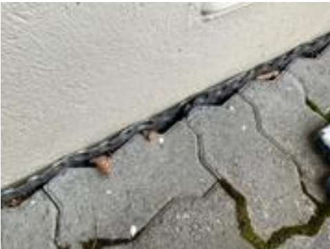
Knotteplasten mangler overgangslist.
