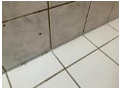
Sprikk/ufagmessige mykfuger i overganger.
