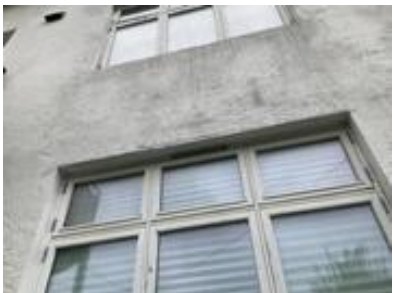
Riss/avskallinger over vindu, her i 1 etg.
