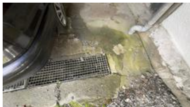
Sprekker i betong
