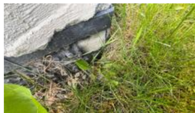
Hull i fuktsperran.
