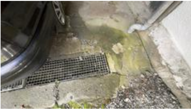
Sprekker i betong
