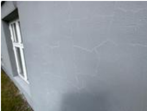
Krakelering i maling/ puss.
