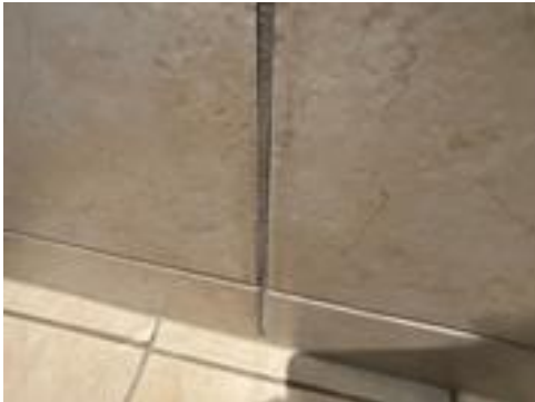
Sprekker i flisfuge.
