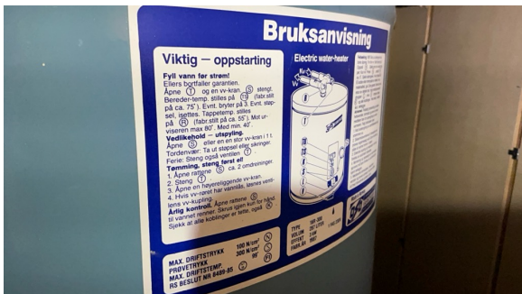
Varmvannstank under trapp.
