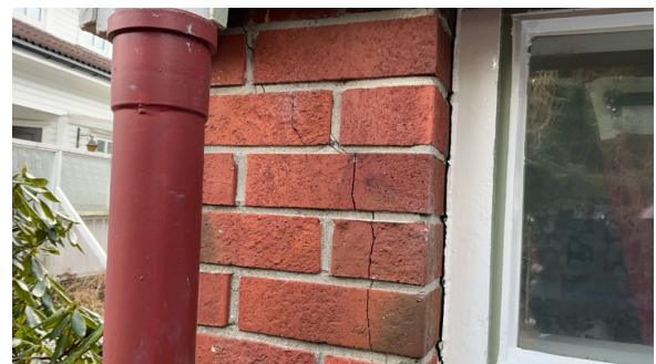
Sprekk i teglsteinsforblending.
