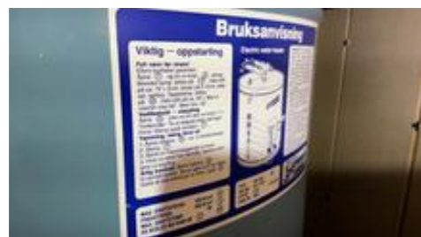
Varmvannstank under trapp.
