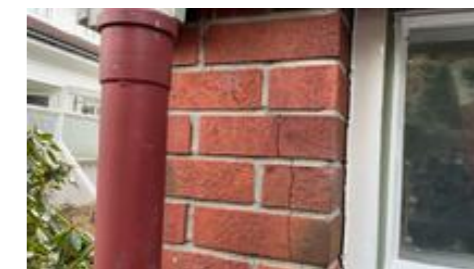
Sprekk i teglsteinsforblending.
