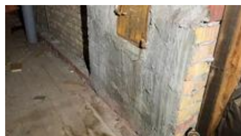
Rust/misfarging under feieluke
