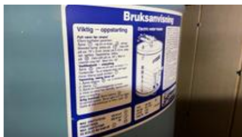
Varmvannstank under trapp.
