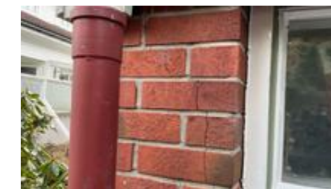
Sprekk i teglsteinsforblending.
