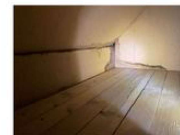
Fuktskjolder i sponplate kneloft.
