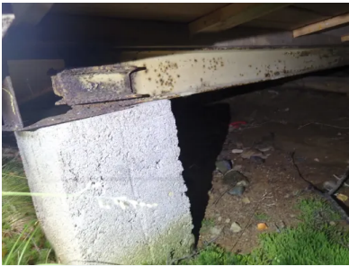
Rust i bjelke.
