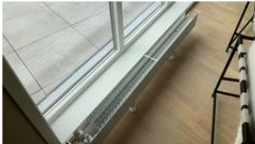
Radiator i stue.
