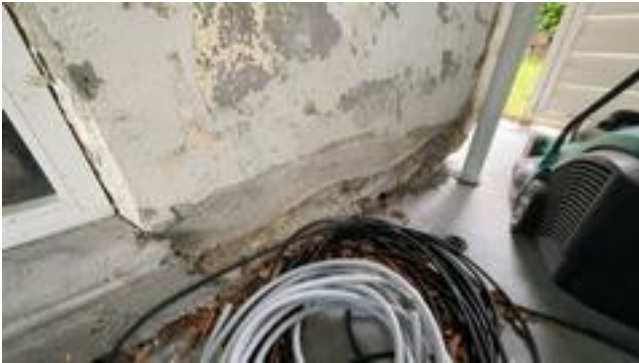
Slitt mur manglende puss observert.
