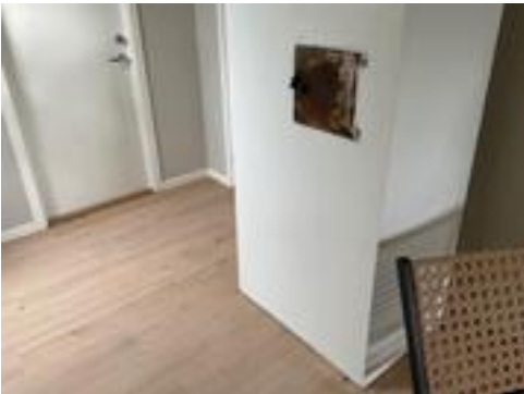
Manglende ildfastplate under feieluke.
