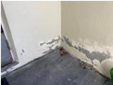
Flassing i maling, pga fukt
