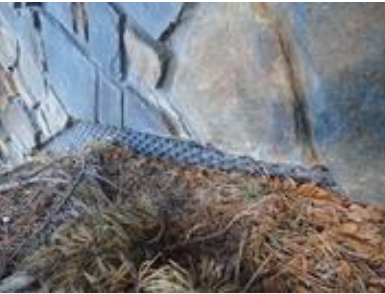
Manglende klemlist over grunnmursplast.
