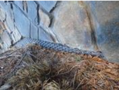
Manglende klemlist over grunnmursplast.
