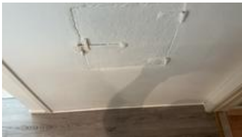
mangler ildfast plate under luker
