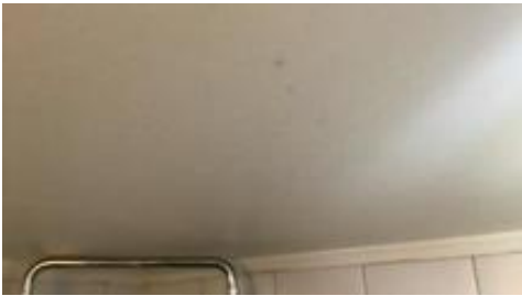
Misfarging i himling.
